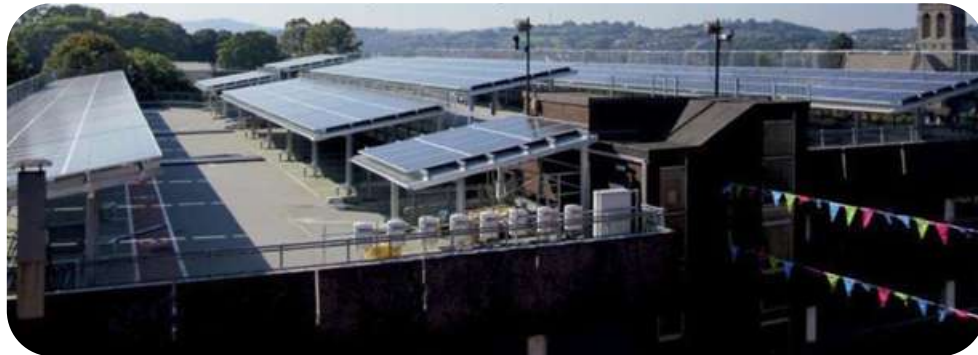
Photovoltaic array installed at Exeter's Mary Arches car park which has provided for a carbon positive building.
